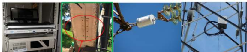
Figure 10 - FBG Interrogator and optics strain and vibration applied at 138 kV tower
