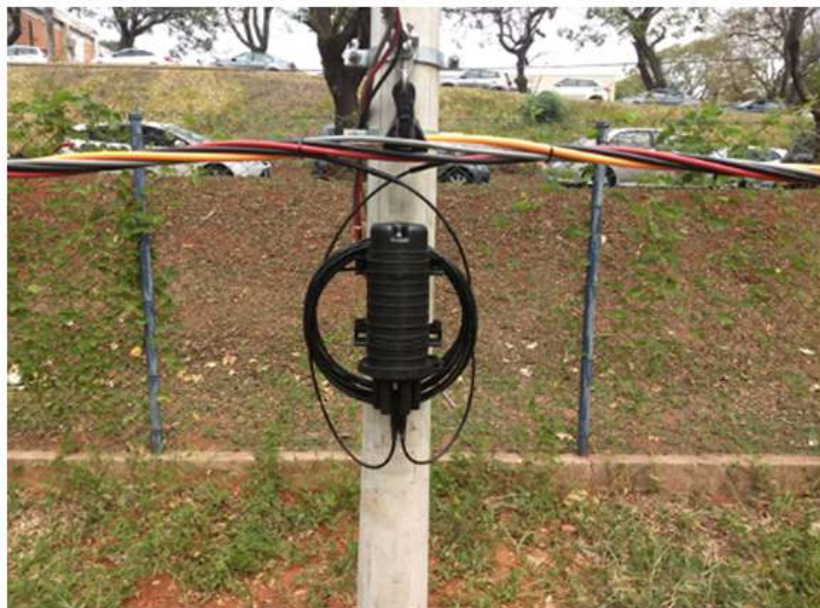
Figure 7 - The optical fiber access of ABC synergic cable in array of low voltage installed on test field of poles
