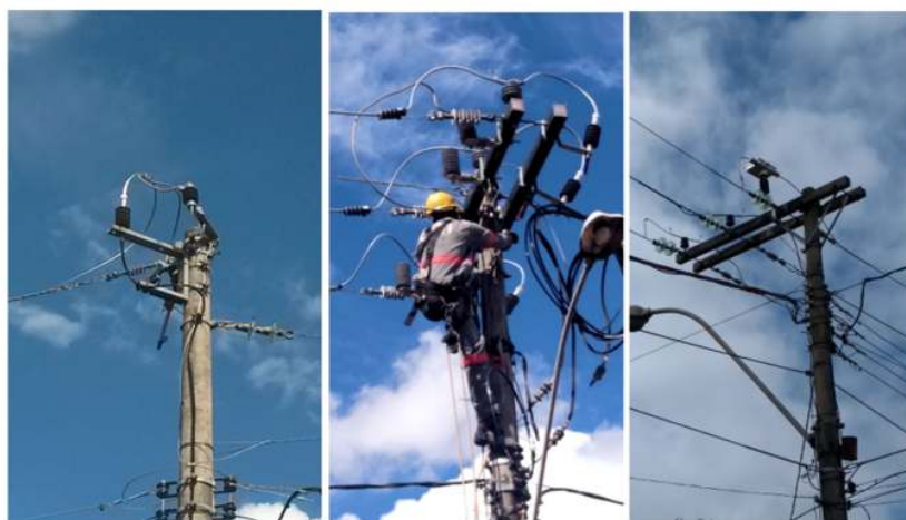
Figure 5 - The termination of optical fibers embedded optical insulator of 13.8 kV (left and center) and setup of fixed on the pole (right)
